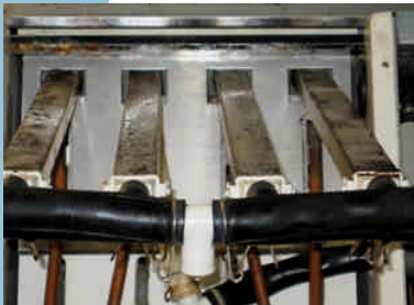
Mold buildup around the water distribution system inside ice machine
